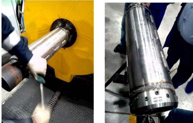
Figure 2—Marker cassette prototype model installation on a branch pipe of a well casing
